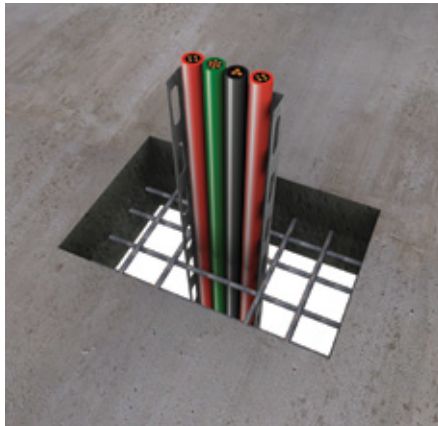
2. For building penetration seals in floors, install 100 mm plugirons. These plug irons should be installed central of mortar penetration seal every 300 mm, but minimum one plug iron on each side and should be inserted 50 mm in the floor and covered by 50 mm of PROMASTOP®-M. No plug irons required for wall application.
